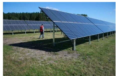
Figure 25: Solar PV in “Minhauzena muiža”
