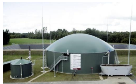
Figure 27: Biogas plant in Farm “Jaundzelves”
