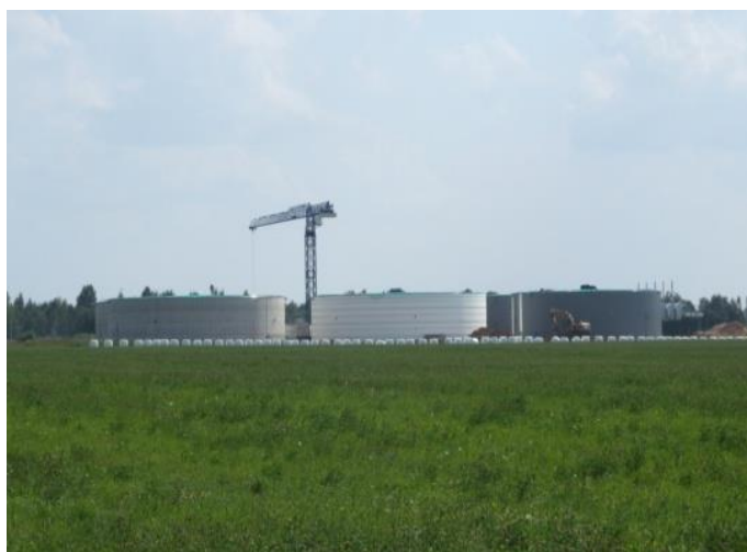
Figure 28: Biogas plant in Farm “Gravas”
