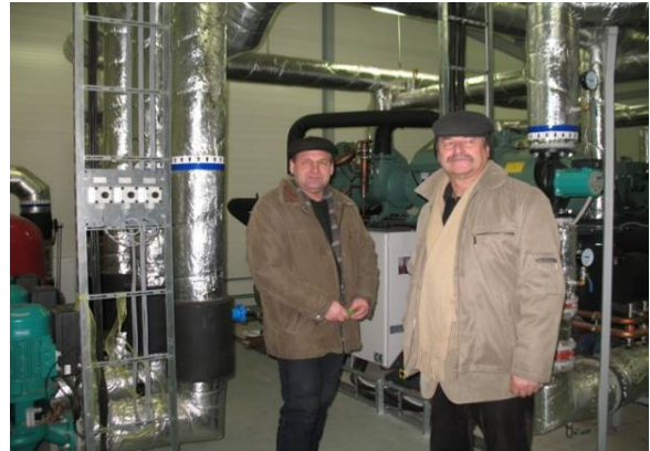
Figure 5.10 Executive director and technical engineer of Salacgriva municipality next to the sea water heat pumps in municipal heating plant
