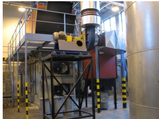
Figure 5 New biomass boiler (1MW H ) in Slavičín
