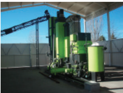
R&D BIOMASS GASIFICATION PLANT (PORTUGAL)
