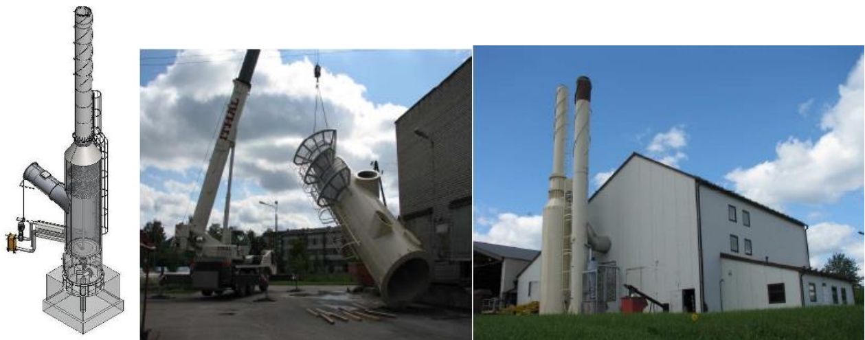
Fig.3. Installation of flue gas condenser in Ludza biomass boiler house in Latvia
