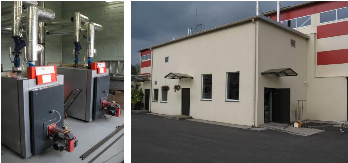
Fig.2. Existing diesel oil boilers and the boiler house
