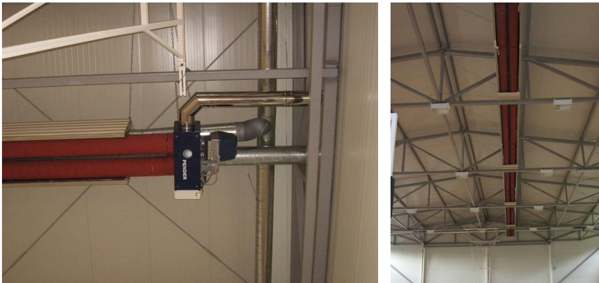
Fig.3. Autonomous heating system in the sports hall
