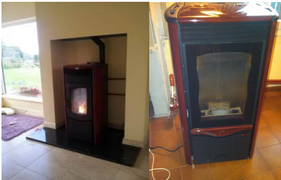
Photo showing typical stove boiler inset into existing fire place.
